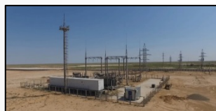
110 kV & 220 kV Substation and PL's Length: PL 110 kV – 38,5 km, PL 220 kV – 42 km Capacity – 12 MW
